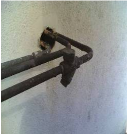
OLD DEFECTIVE STEAM TRAP
