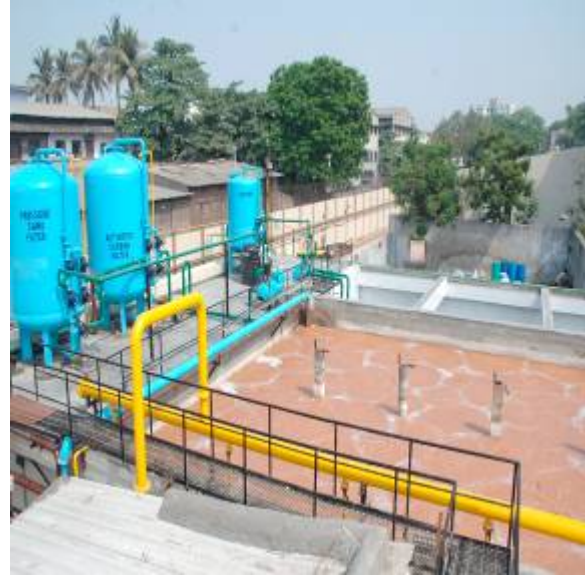
Carbon Filter, Sand Filter & Softener
