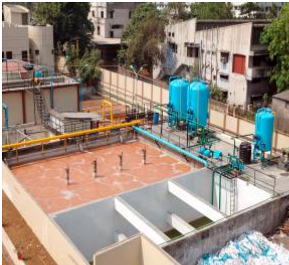
Top view of complete ETP with all units
