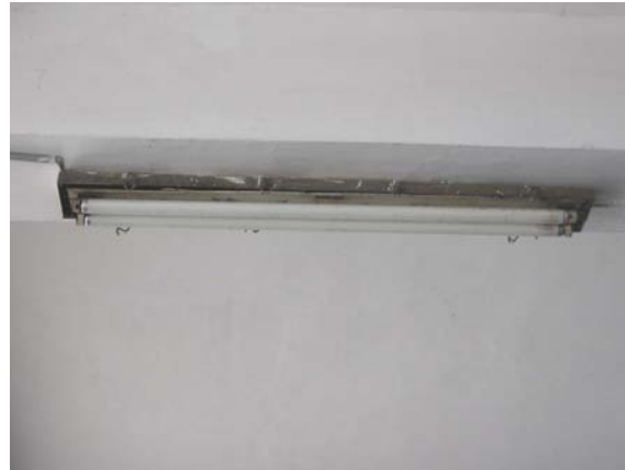
Old Less energy efficient Tube lights
