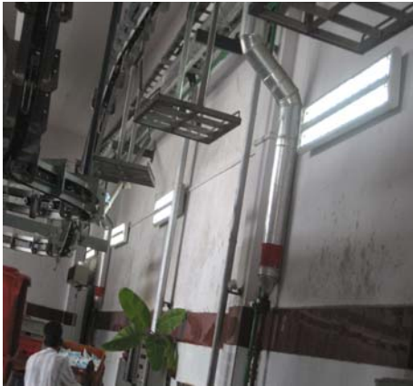
New Energy Efficient Tube lights
