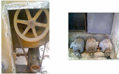
7.5 Hp Blower motor
