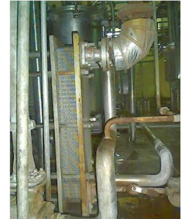
PHE SYSTEM IN NEW MILK PASTEURISER
