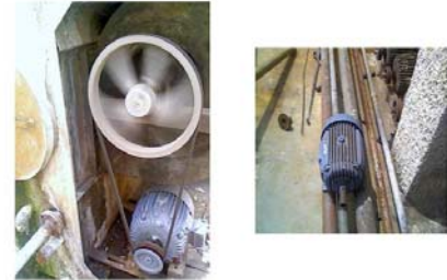
5 Hp Blower motor
