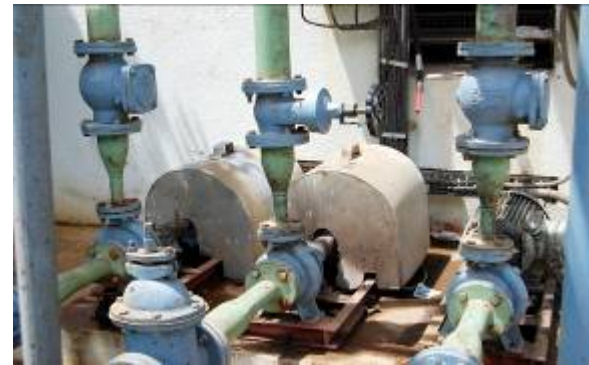
Cooling water pumps
