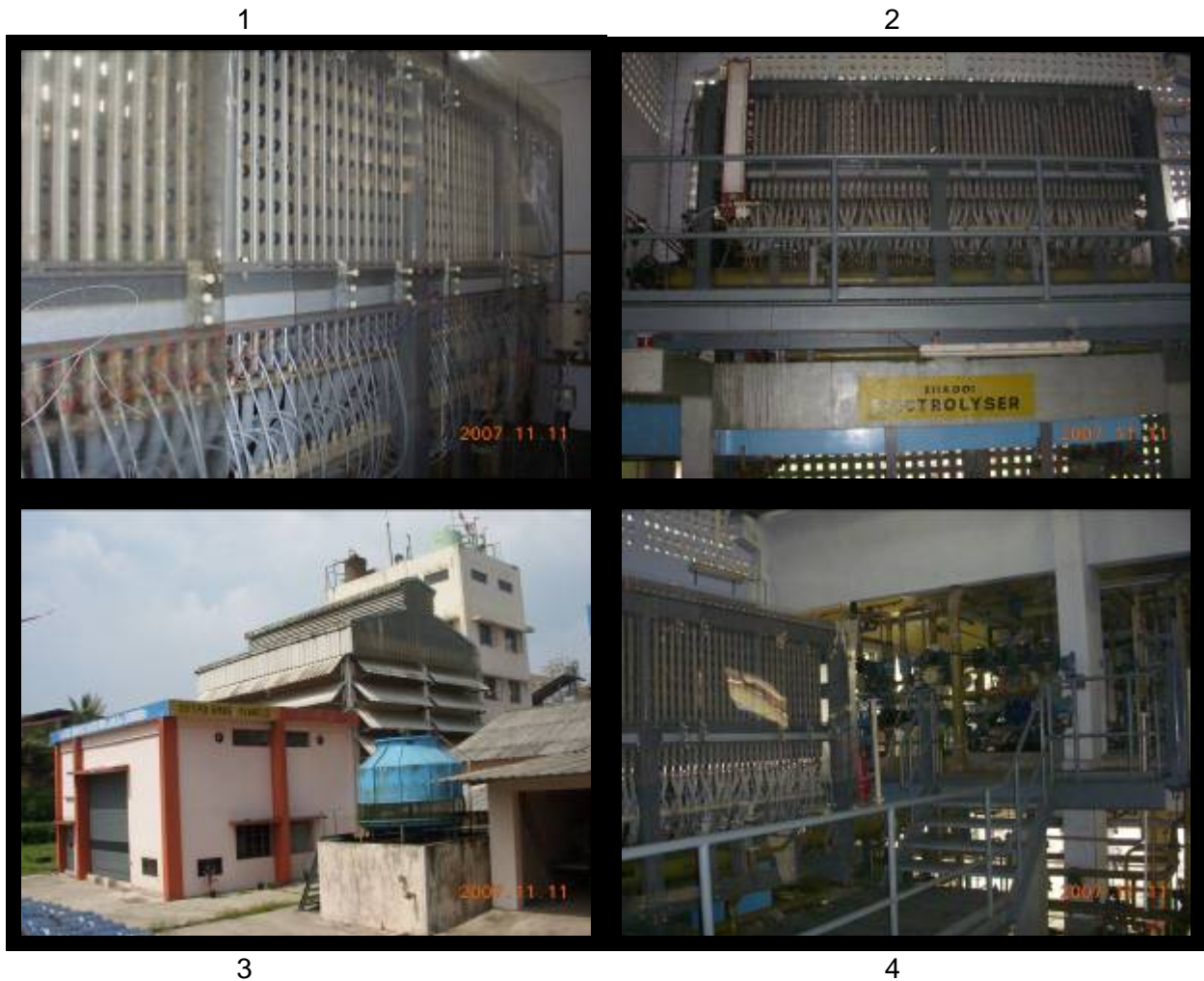
Fig: 1, 2, 3, 4. – 25 TPD MEMBRANE CELL PLANT – PHASE III
