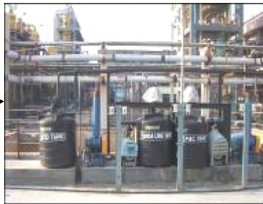
Chemical dosing system
