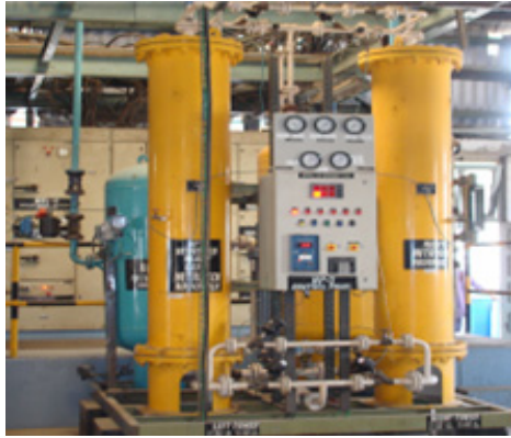
New Nitrogen Generation Plant
