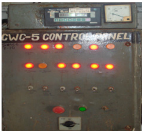
Temperature Controller for Chilled Water Compressor
