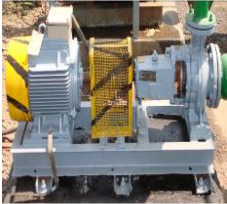
New High Efficiency Mega-G-65/160 Pump with EFF1 20 HP Motor
