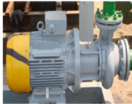
New High Efficiency Grundfos Pump with EFF1 20 HP Motor
