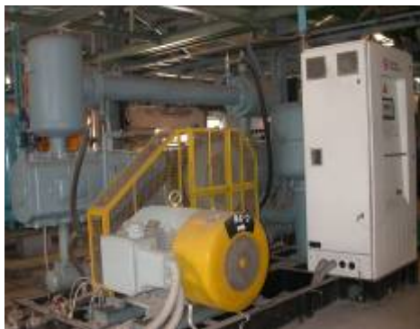
New Air Compressor With VFD System
