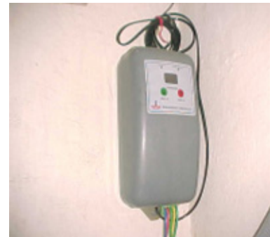
Temp sensors for AW
