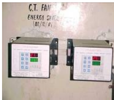
Temp. sensor Cooling tower
