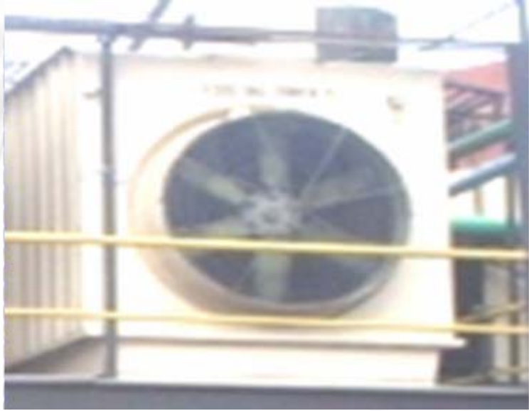
Electric driven cooling tower Energy cost- Rs. 3.60 Lacs/annum
