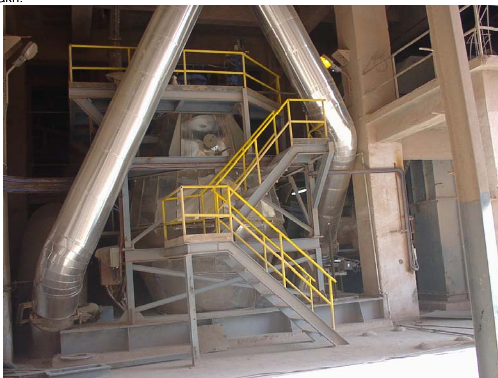
Dynamic Separator at Raw Mill
