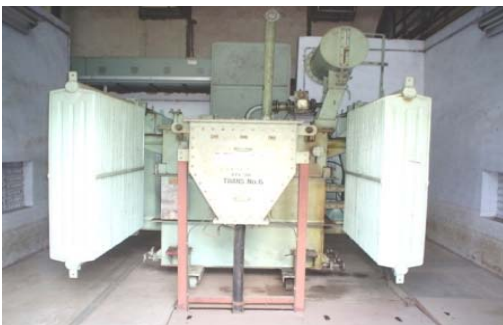
Before –Oil type transformer
