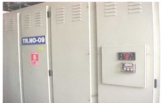
After :Unitize substation with dry type transformer
