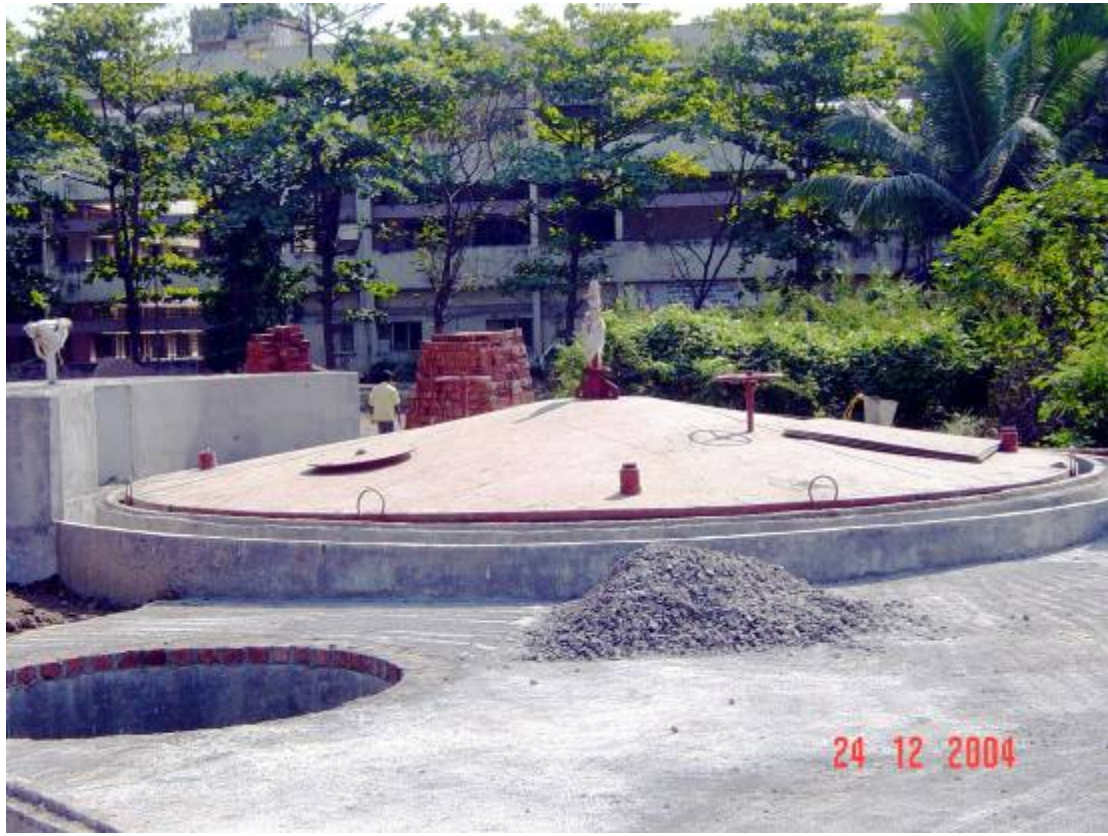
METHANE GAS PLANT FROM BIODEGRADABLE WASTE
