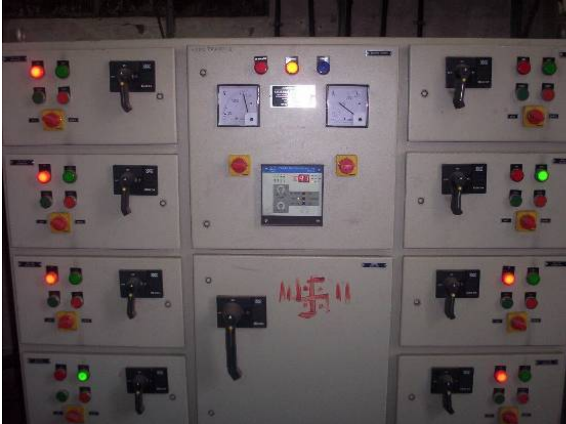
AUTOMATIC POWER FACTOR CORRECTION PANEL
