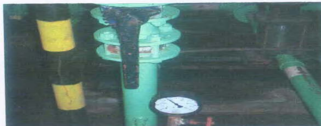
VALVE IN FULL OPEN CONDITION
