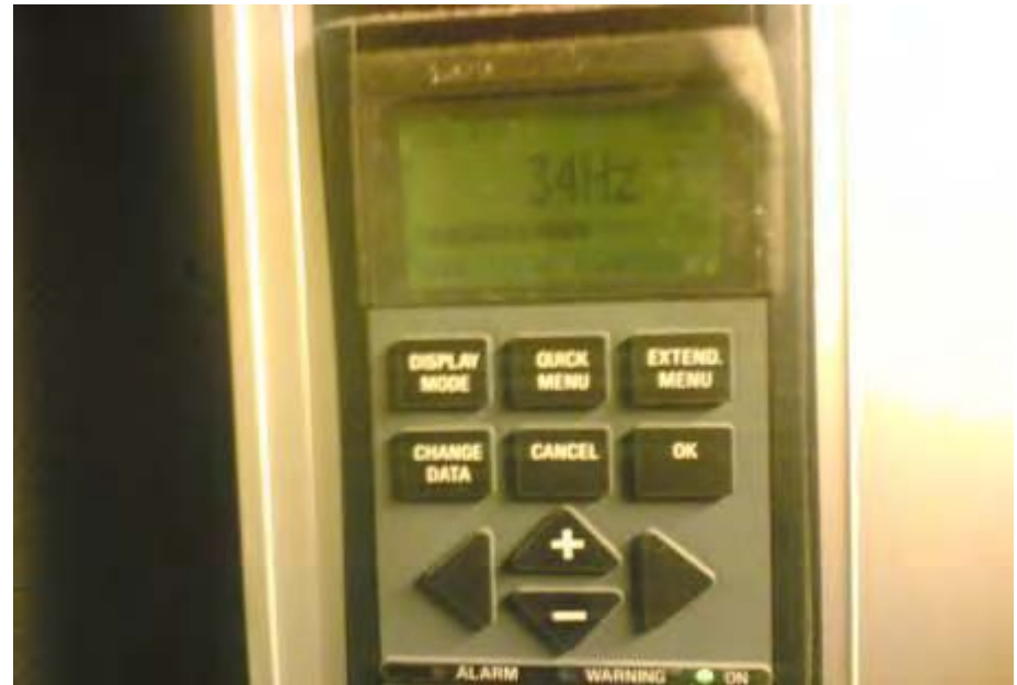
Display signifying the modulation of speed of the VFD depending upon the load
