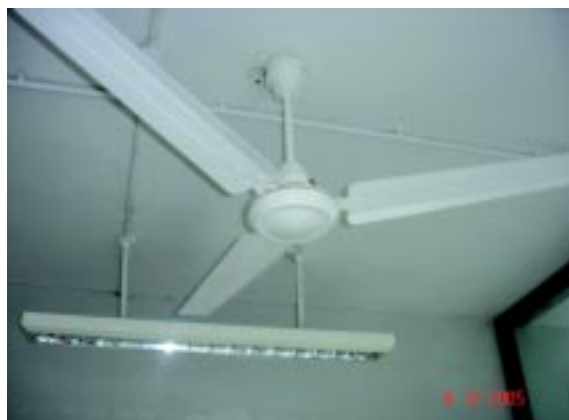
Ceiling fans consuming less energy installed
