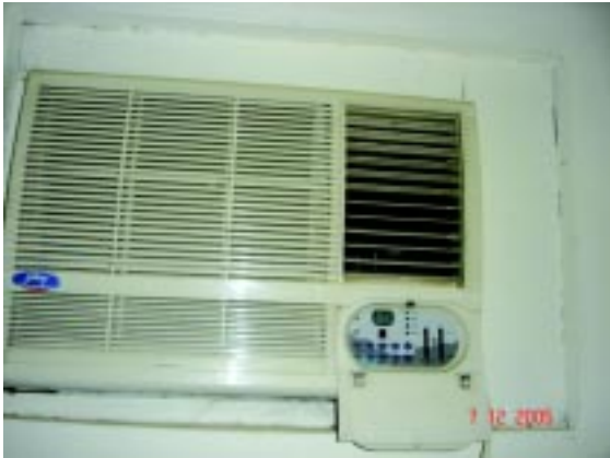
Digital remote controllers provided in window AC units
