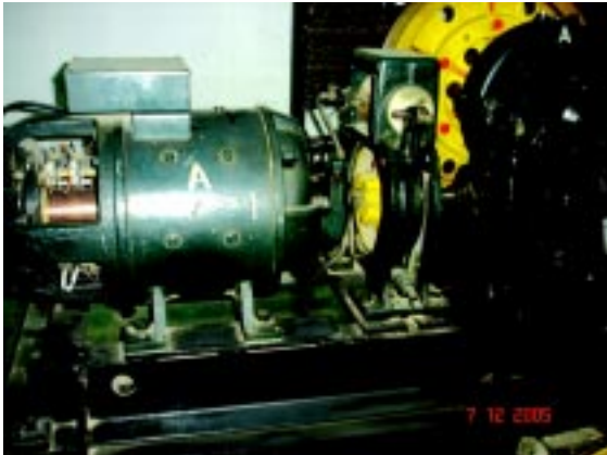
Old DC drive Lifts 11 KW - Replaced
