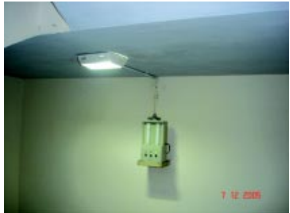
2x11 W energy saver fitting installed in all stairs and lobby
