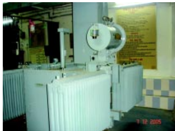
After office hours and on holidays one transformer is switched off to save energy
