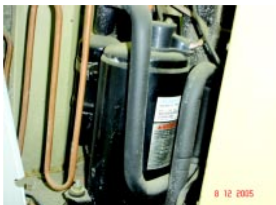
Energy saver Rotary compressors installed
