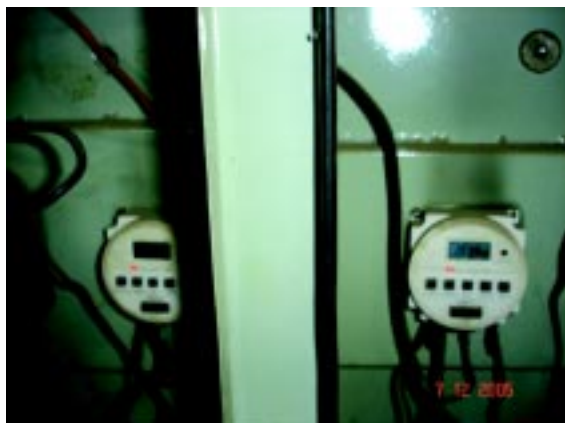
Timers provided to switch off At mid-night half of the compound light to save energy
