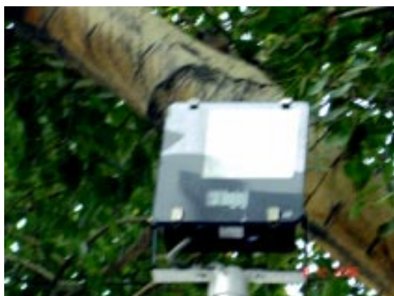
250 W metal halide lamps installed
