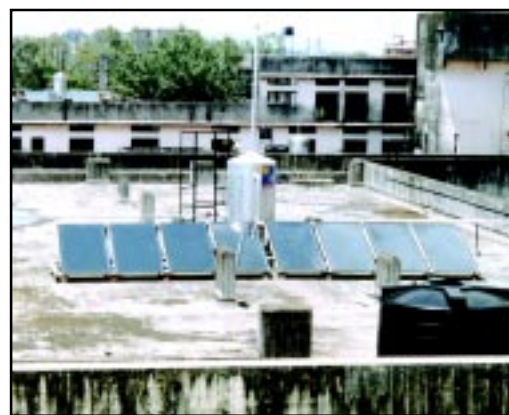
SOLAR WATER HEATING SYSTEM (TOTAL 19050 LPD)
