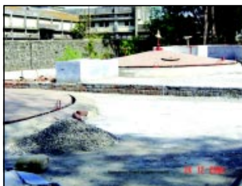
METHANE GAS PLANT FROM BIODEGRADABLE WASTE
