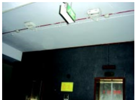
2x11 W energy saver fitting installed in all lift lobbies
