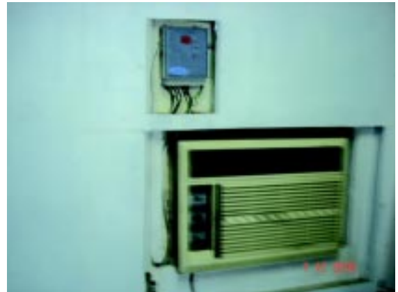
Smart controller provided for selective / sequential operation of AC units
