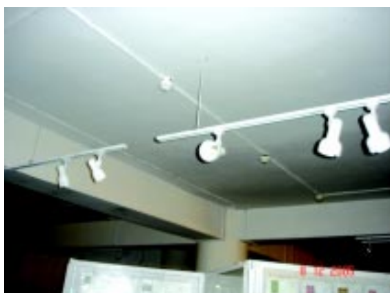
8W CFL lamps in Philatelic Museum installed
