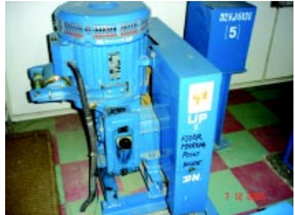
New VVVF AC Drive Lifts of 5 KW Installed. Power saved 6 KW / lift
