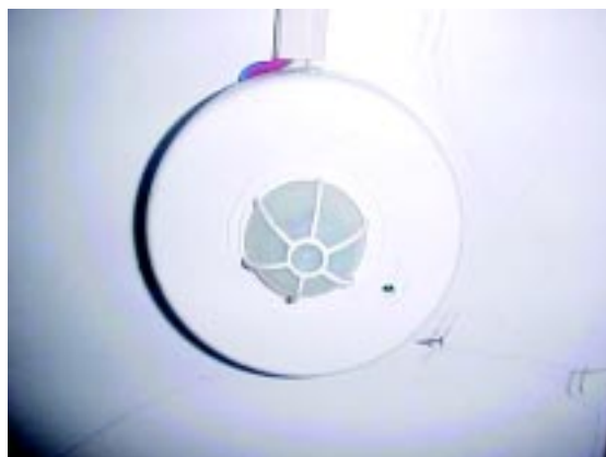
Occupancy Sensor Installed in Cabin
