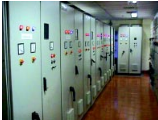
VFD PANELS FOR ID AND FD FANS OF 100TPH BOILERS
