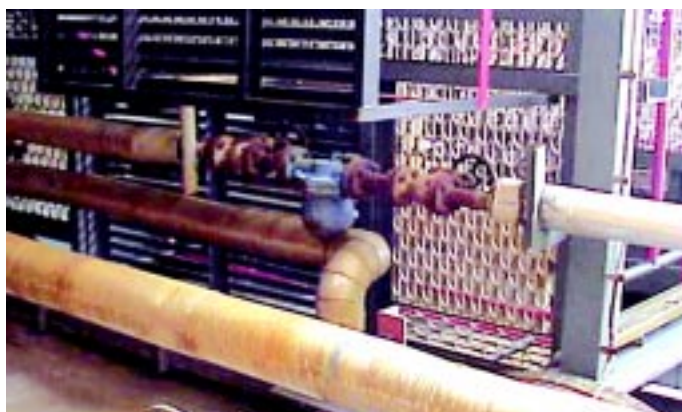
Float Type Steam Trap in Boiler IV SCAP Outlet Line
