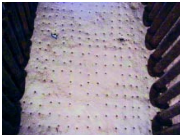
Ceramic Insulation Inside 31-F-01 Furnace
