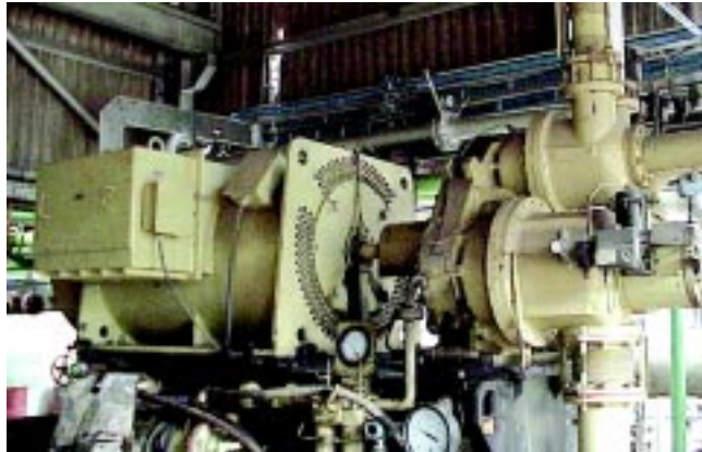
New Centrifugal Air Compressor
