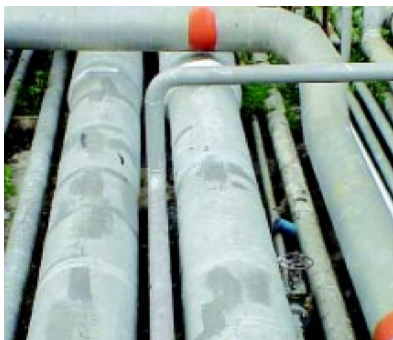
Calcium Silicate Insulation Over Steam Header
