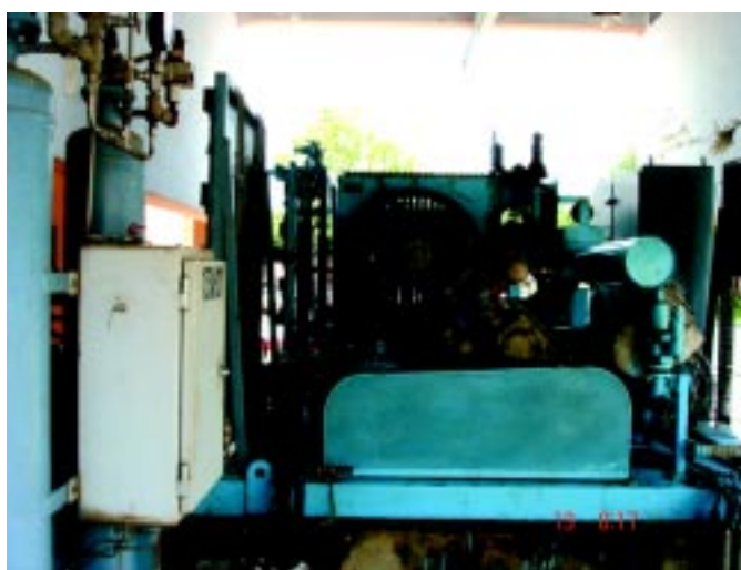
IA COMPRESSOR STOPPED
