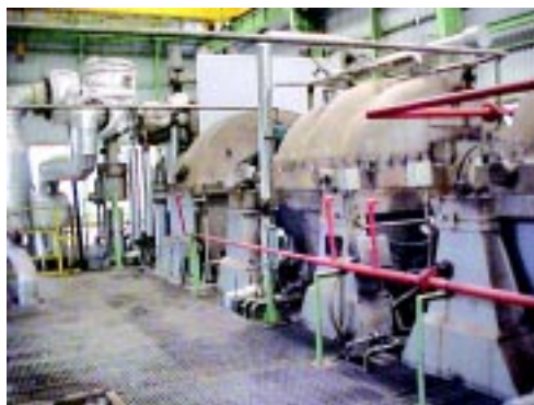
Cracked Gas Compressor
