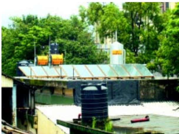
Solar Hot water heating system
