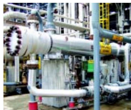
Process - Process Exchanger - PE Plant
