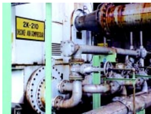
Decoke Air compressor
