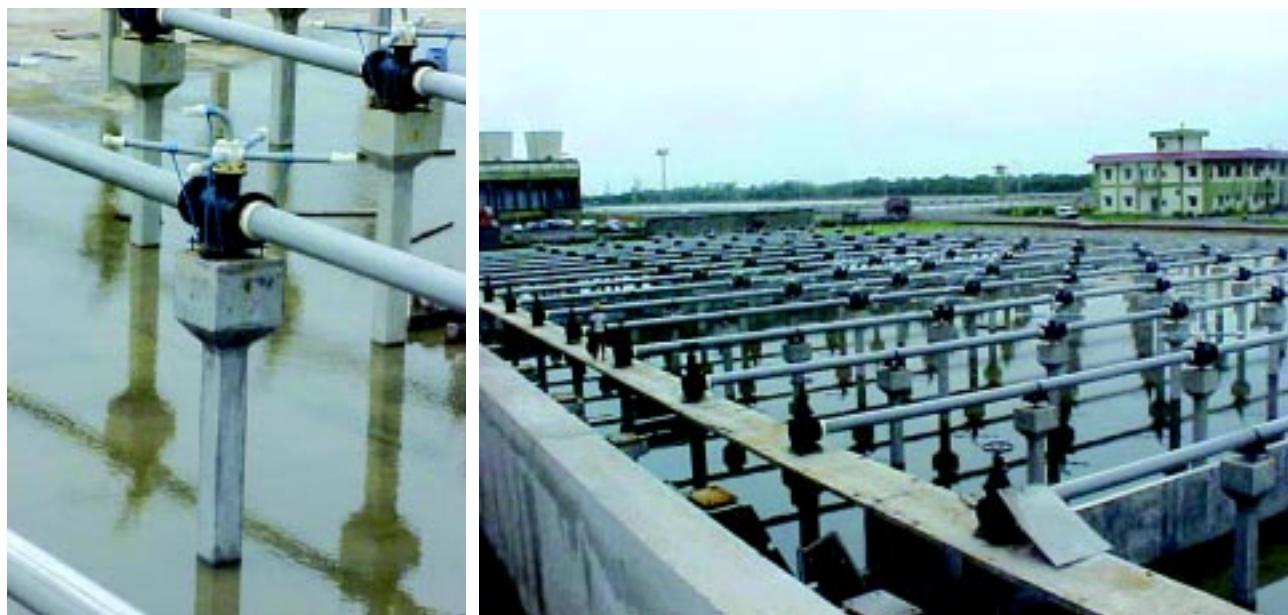
Mist Cooling Pond & Spray nozzle.
