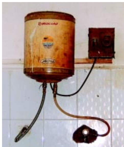
Electrical heating for canteen hot water
