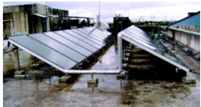
Solar water heater for preheated water inlet to Steamer.
