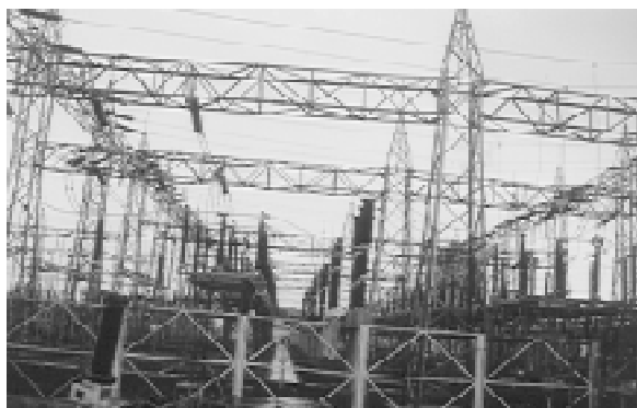
MRS installation for stabilization of power supply
