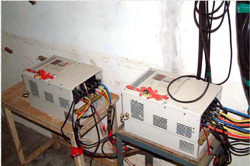
V.F.D for Chlorine Blowers
