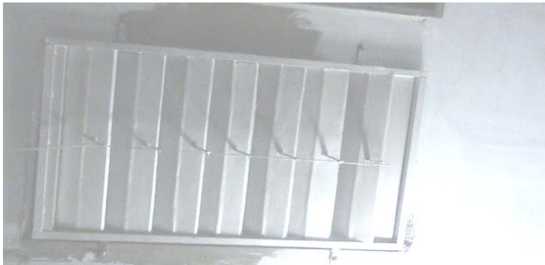
ADDITIONAL FRESH AIR DAMPERS FABRICATED INHOUSE FOR IMPROVING FAN EFFICIENCY
