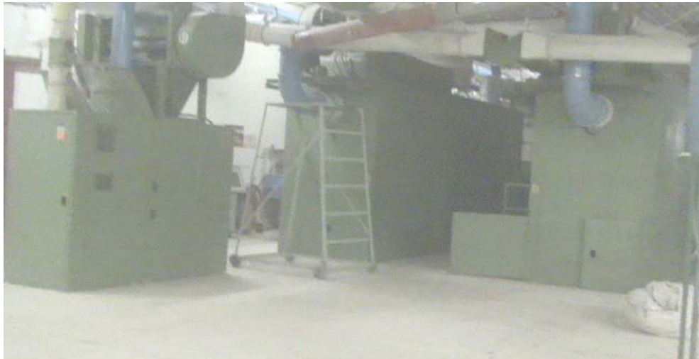
TWO LINES RUNNING WITH ONE NO. VARIO CLEAN IN UNIT NO2
