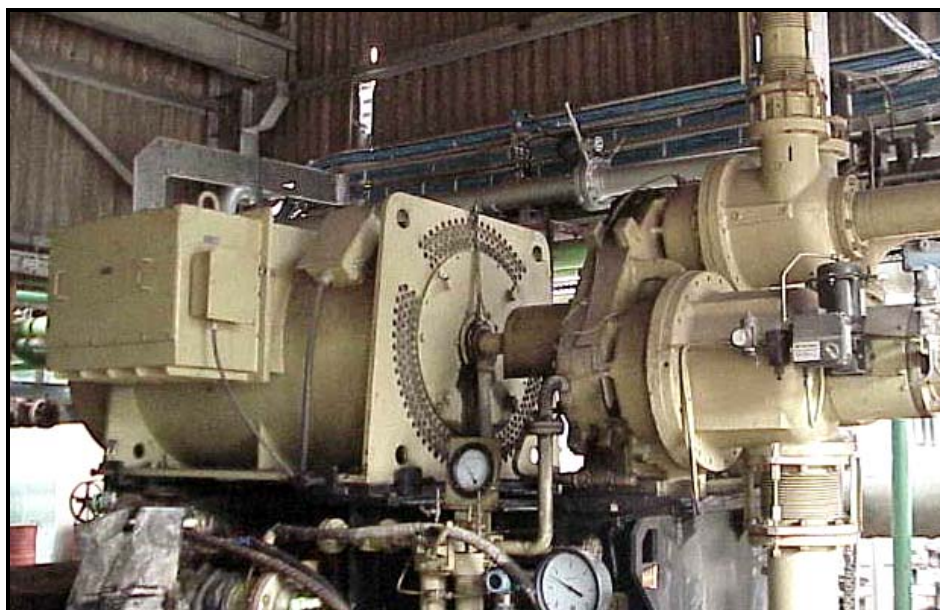
New Centrifugal Air Compressor
