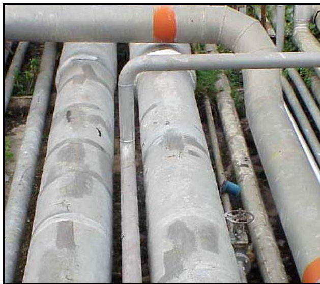
Calcium Silicate Insulation Over Steam Header
