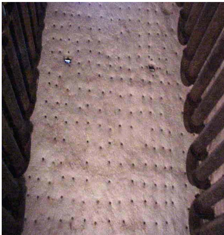
Ceramic Insulation Inside 31-F-01 Furnace
