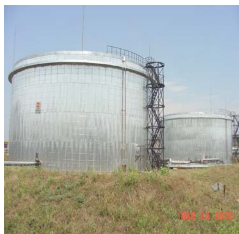
Tanks after Insulation
