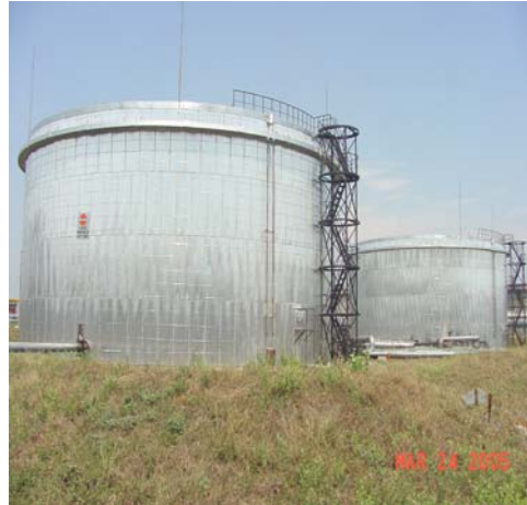
Tanks after Insulation
