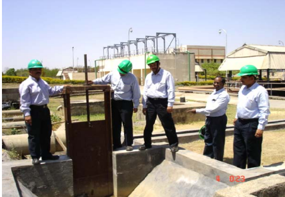
PROVIDING SLUICE GATE ON STORM WATER DRAIN TO UTILIZE IT FOR HORTICULTURE
