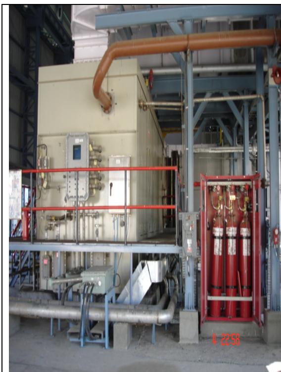
Solar Gas Turbine Compressor
