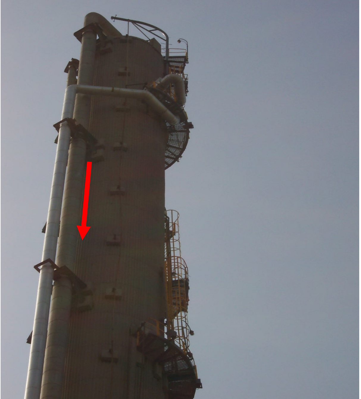
Ethylene Tower Vapor Feed To VCM
