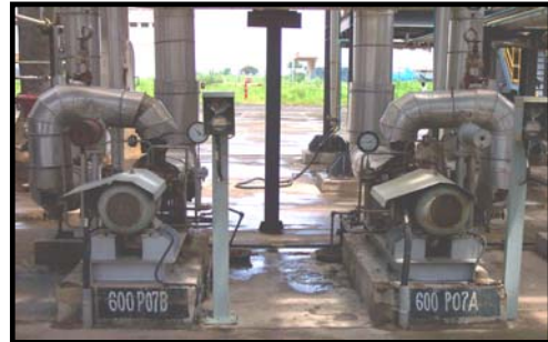
Product Stripper bottom pumps having trimmed impellers (600 P-7 A/B)
