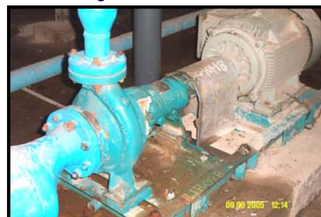
New Raw water Pump (P-1807 A/B)
