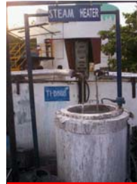
Steam Coil Heating
