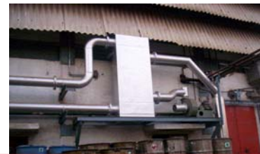
Waste Heat Recovery Heat Exchanger
