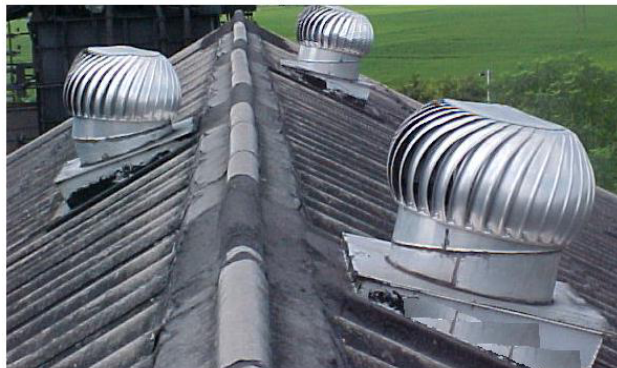
NATURAL VENTILLATORS VIEW FROM ROOF
