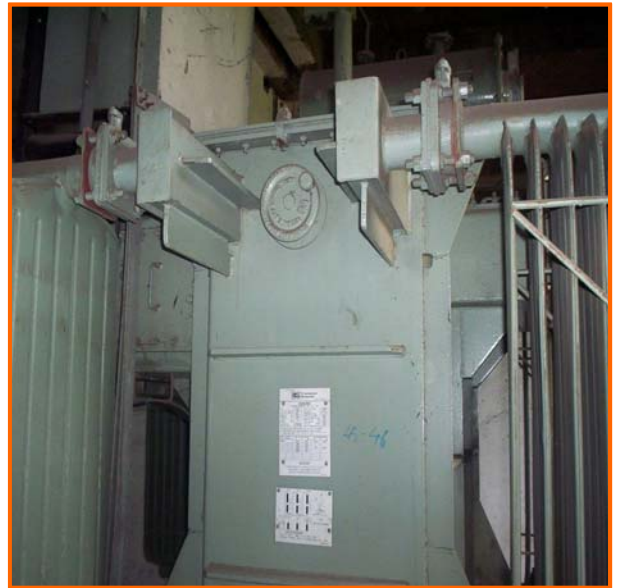
Transformer Tap position
