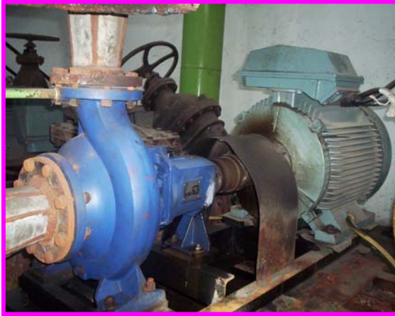
New 75 KW, 245 m3/ Hr capacity Pump
