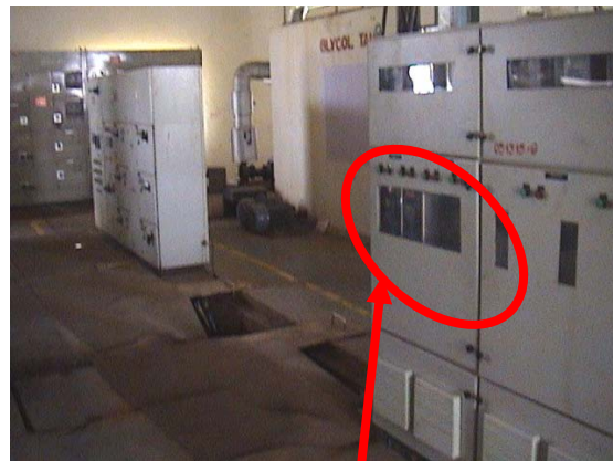
VFD Panel in Chilling Plant
