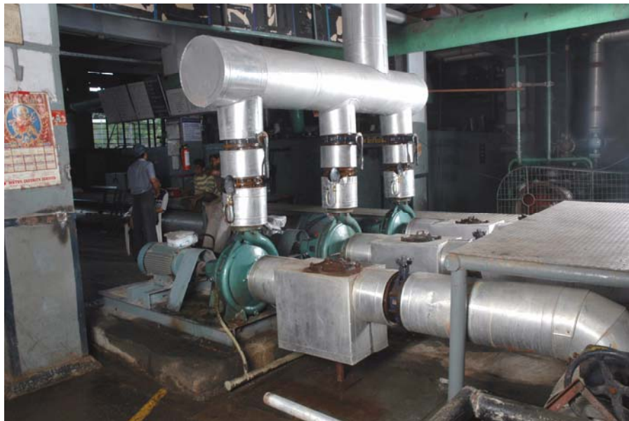
Chilled Water Pumps and header system
