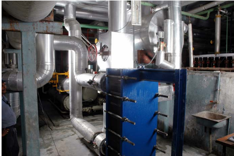
Ammonia PHE with Accumulator (-2 deg C)
