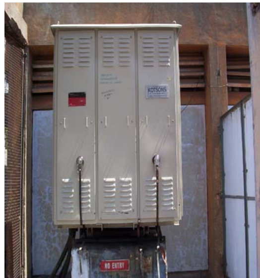
New Dry Type Transformer (99.3% efficiency)
