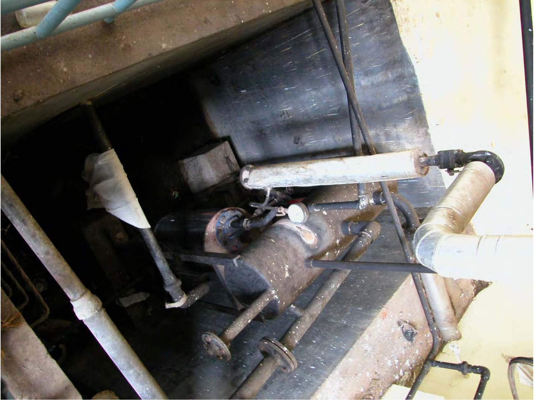
Pressure Powered Pump at Kashayam Plant
