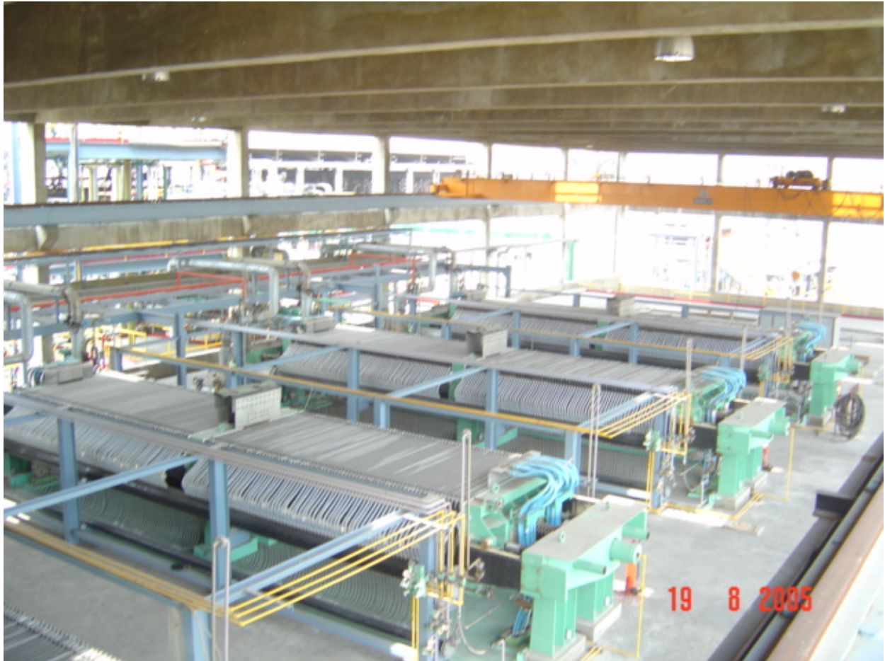
Picture: Electrolyser area
