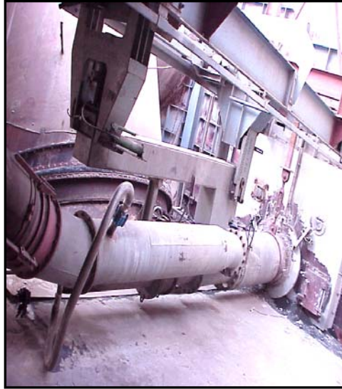
Fig. View of Inlet to Duo-Flex Burner in Kiln-I
