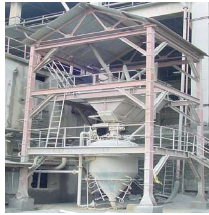
Dry Fly Ash Pumping
