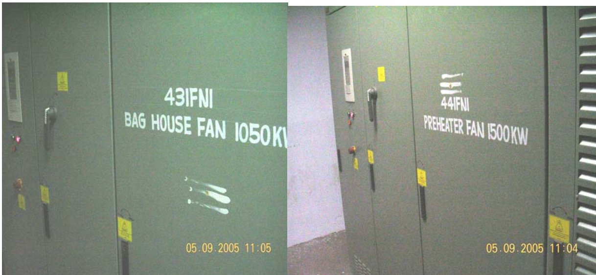
Variable frequency drive for Bag House Fan and Pre-heater fan
