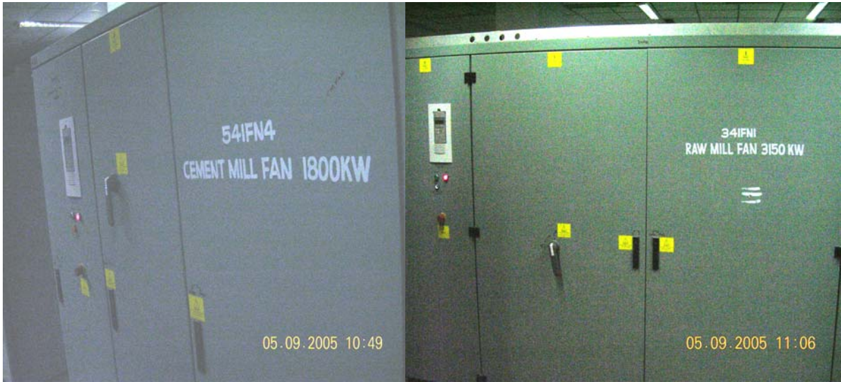
Variable Frequency Drive for Cement Mill fan and Raw Mill fan
