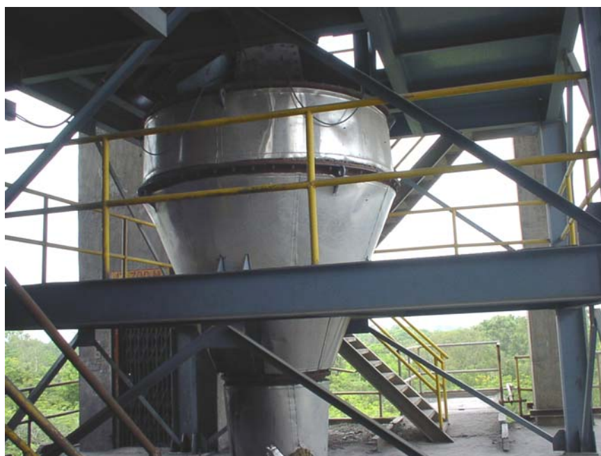
Dynamic Separator Installed in Coal Mills
