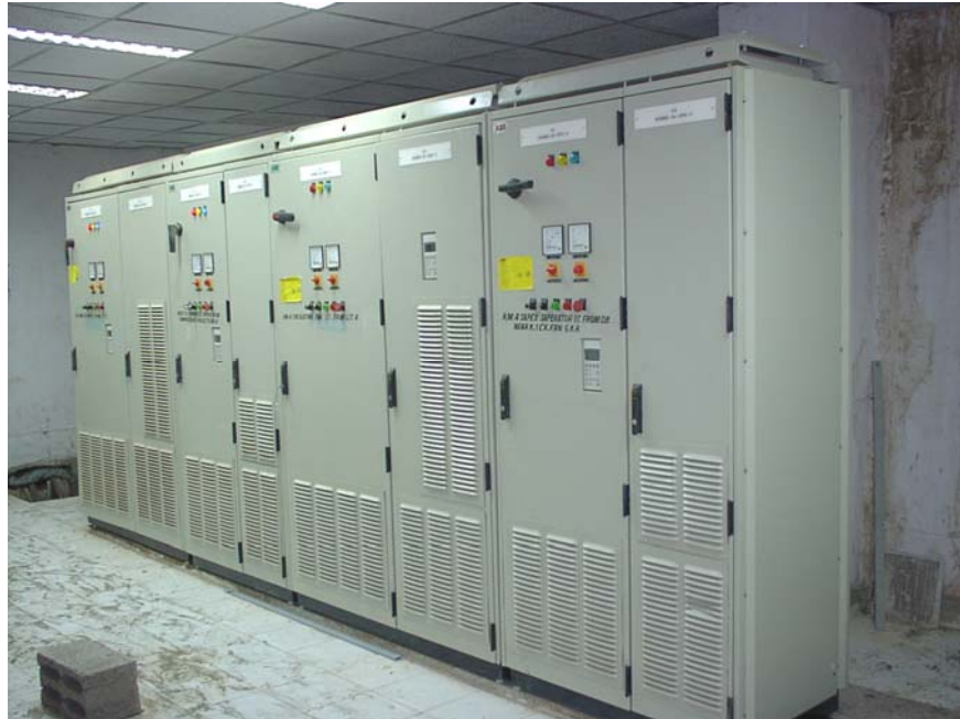
VVVF panels installed at various process fan drive
