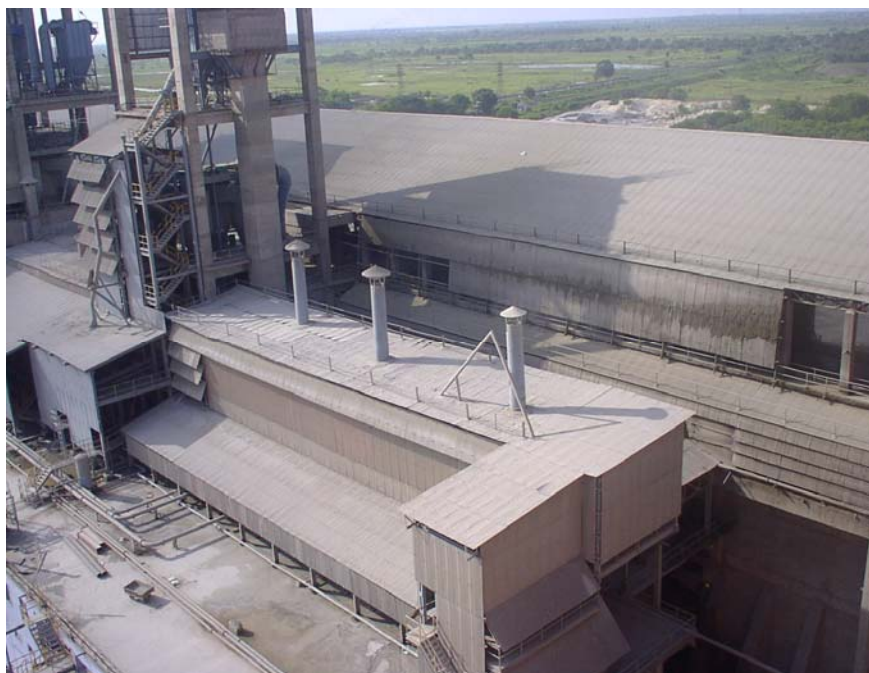
Smokeless chimneys of cement mills
