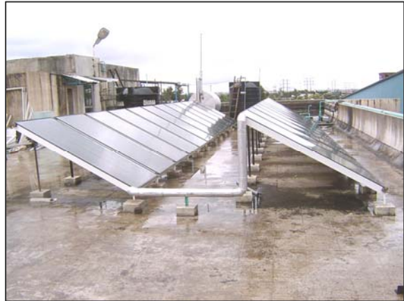
Solar water heater for preheated water inlet to Steamer.
