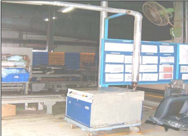
Electrical heating for generation of steam
