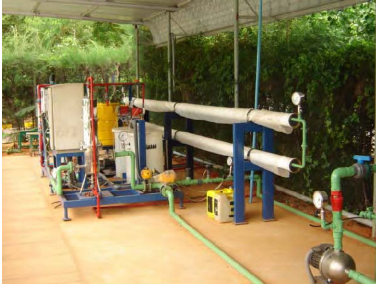
Reverse osmosis plant for Effluent recycling – Water Conservation
