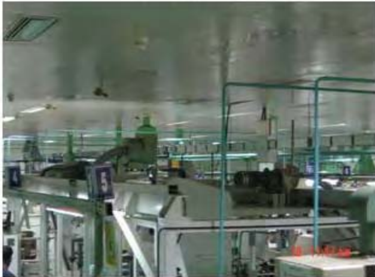
INDIVIDUAL FUME EXTRACTION UNITS
