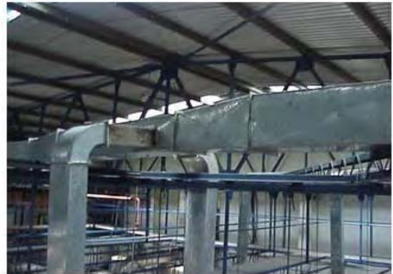
A COMMON DUCT CONNECTING INDIVIDUAL FUME EXTRACTION UNITS
