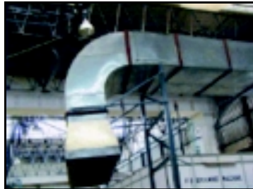
Exhaust system for PU cushion machine
