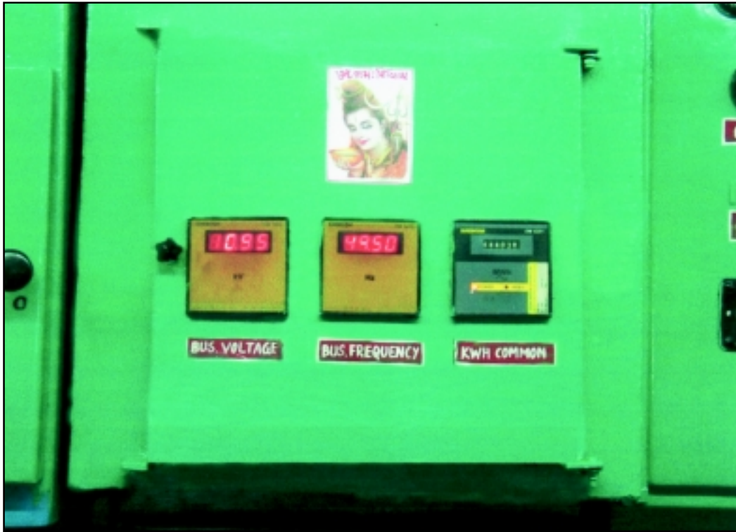
Frequency reduction of Power Generation from 50 Hz to 49.5 HZ
