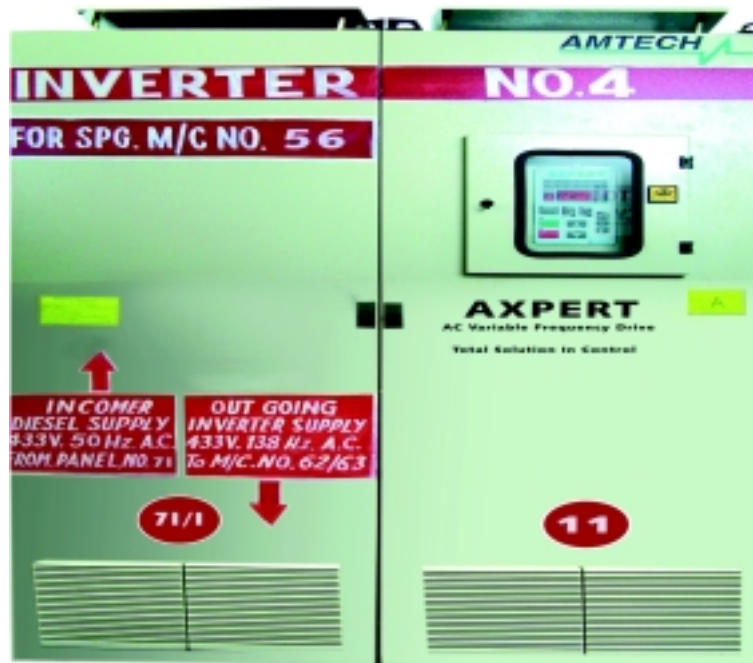
Energy conservation and reduction of product rejection using Variable Frequency Drive
