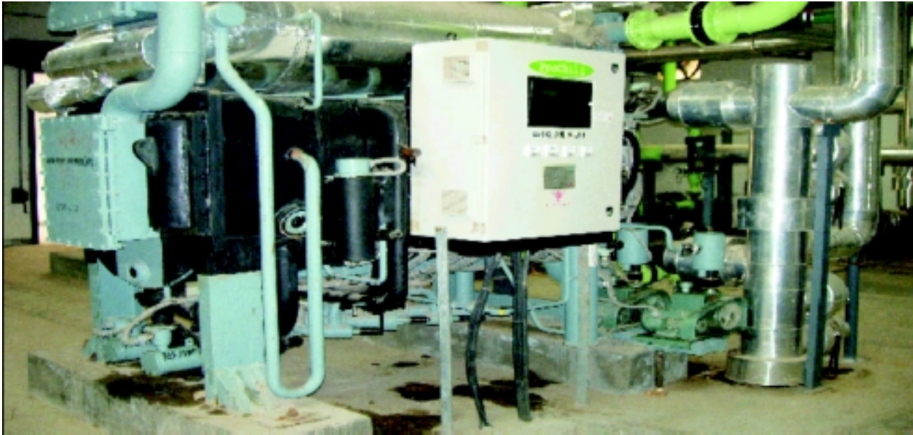
VAM (VAPOUR ABSORBTION MACHINE) INSTALLED AS AN ENERGY CONSERVATION MEASURE , POWER SAVED : 940 KW /YEAR
