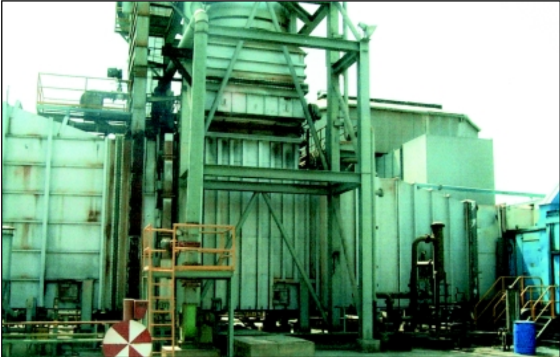
Gas Turbine Bypass Stack Damper Double Sealing
