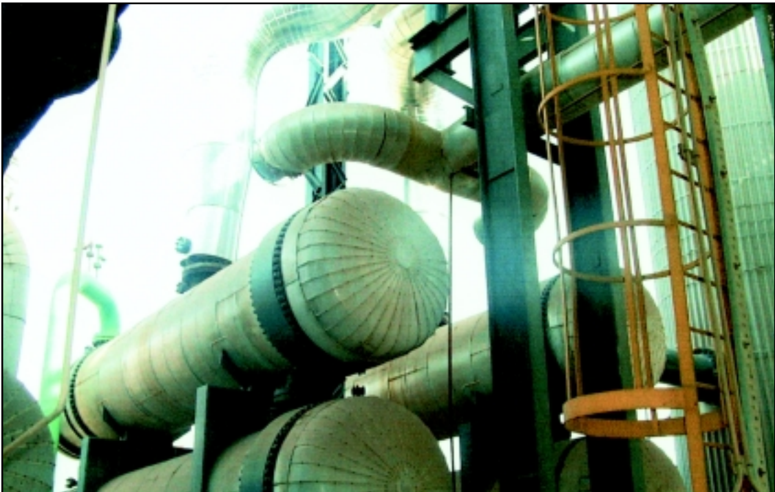
CGC Discharge Line Modification for Power saving
