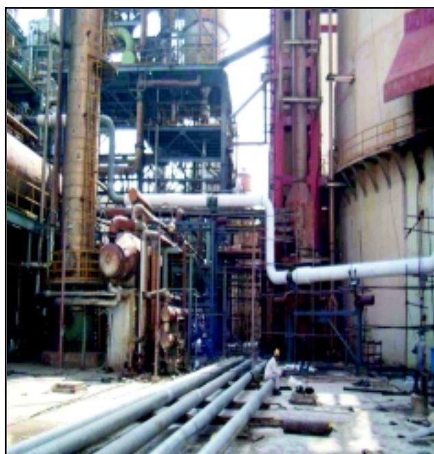
NEW HIGH PRESSURE STEAM HEADER FOR TG SETS
