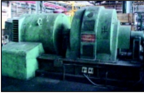
MG Set for 1000 HP Motor Eliminated
