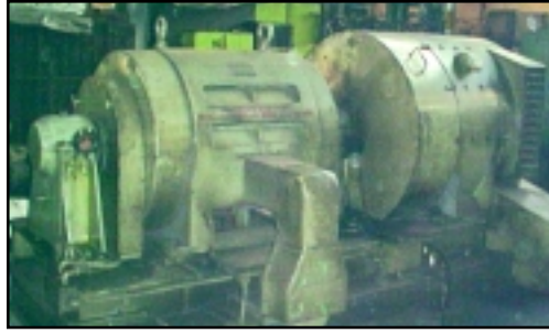
MG Set for 400 HP Motor Eliminated
