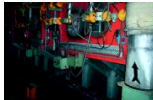
Coal Gas System at Preheater
