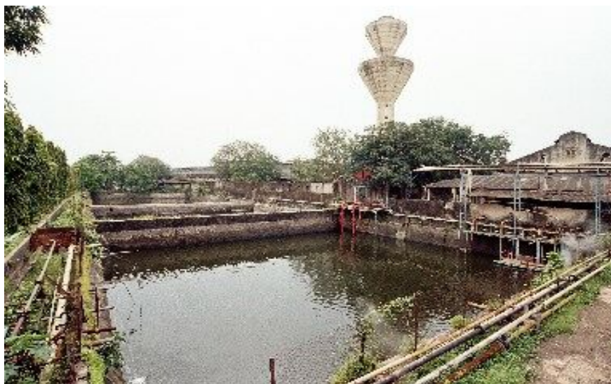
Cleaning of water reservoir tanks resulted in reduction of load on the water softening plant and subsequent saving in pump motor
