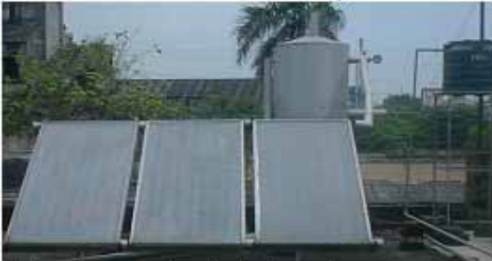
Solar System installed above Canteen.
